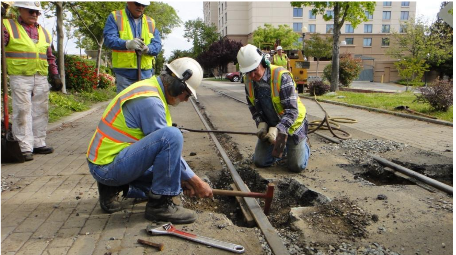
With the impact wrench striking out, Alan and Steve use a track chisel in a futile attempt to break the nut off the bolt
