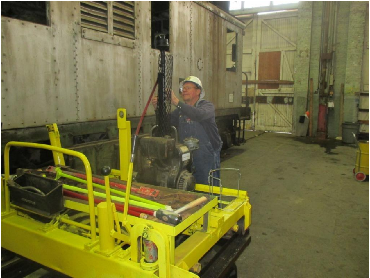
Cliff installs the shield on the new exhaust pipe that Alan built
