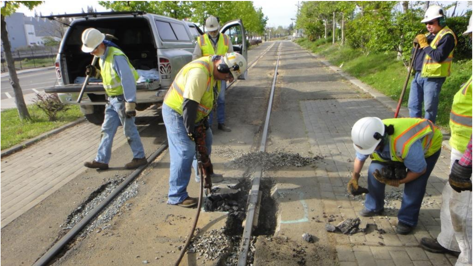
Pam picks-up asphalt debris as Mike F. with the jackhammer cuts around the joint
