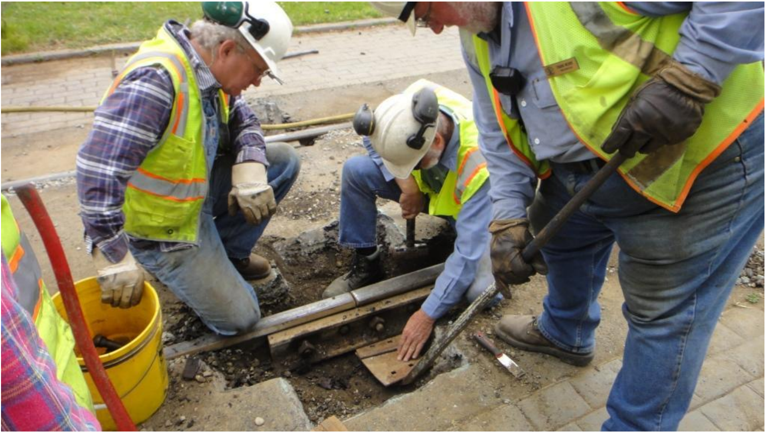
Steve, Alan, and Frank insert tie-plates between the base of the joint-bars and the sunken tie to add stability and support
