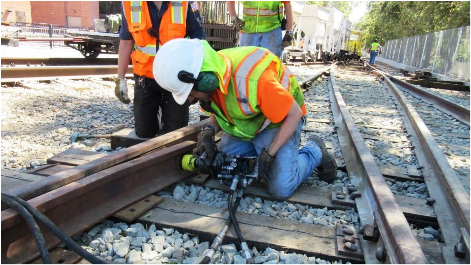
With everything now fitting together, Matt uses the hydraulic impact wrench to tighten down the bolts
