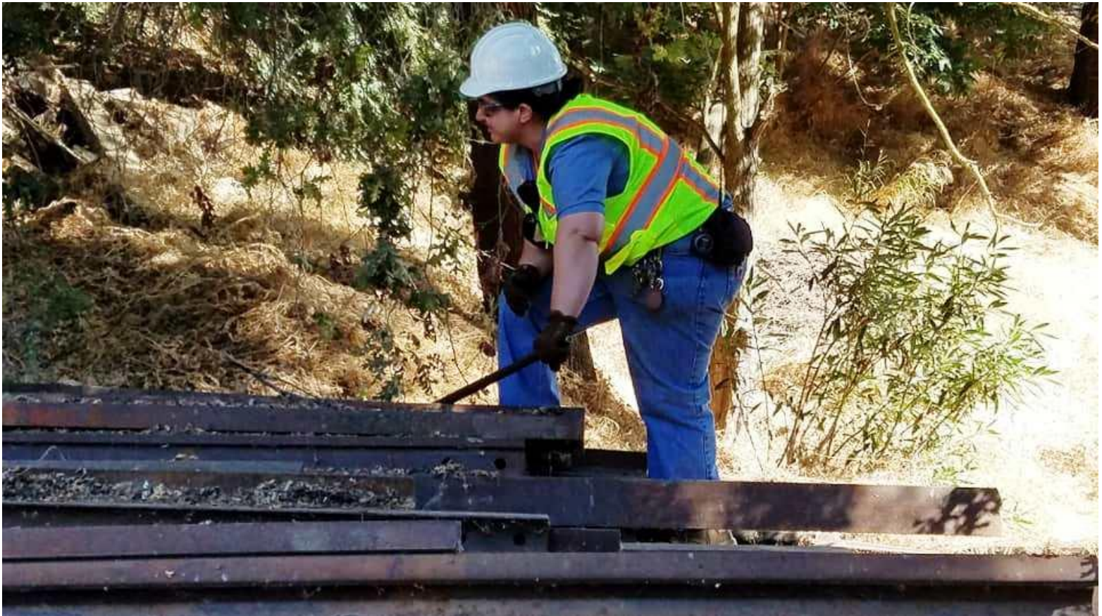
Heather, using a rail-fork, rolls the next stick of rail so that the rail-tongs can grab it
