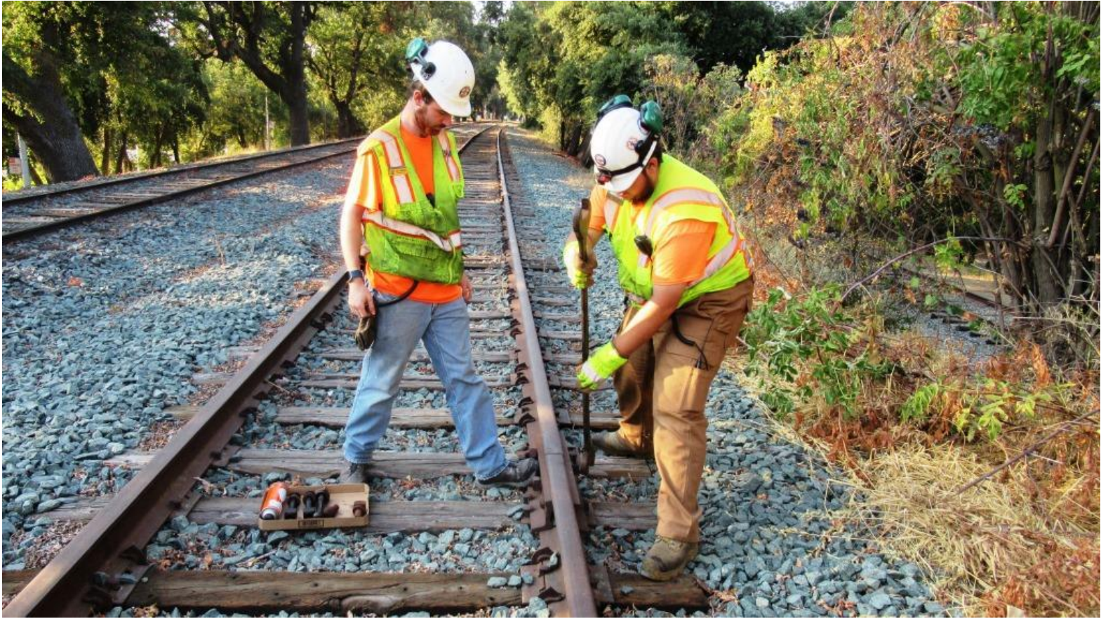
Matt and Chris replace a broken bolt on the Miller Park Siding
