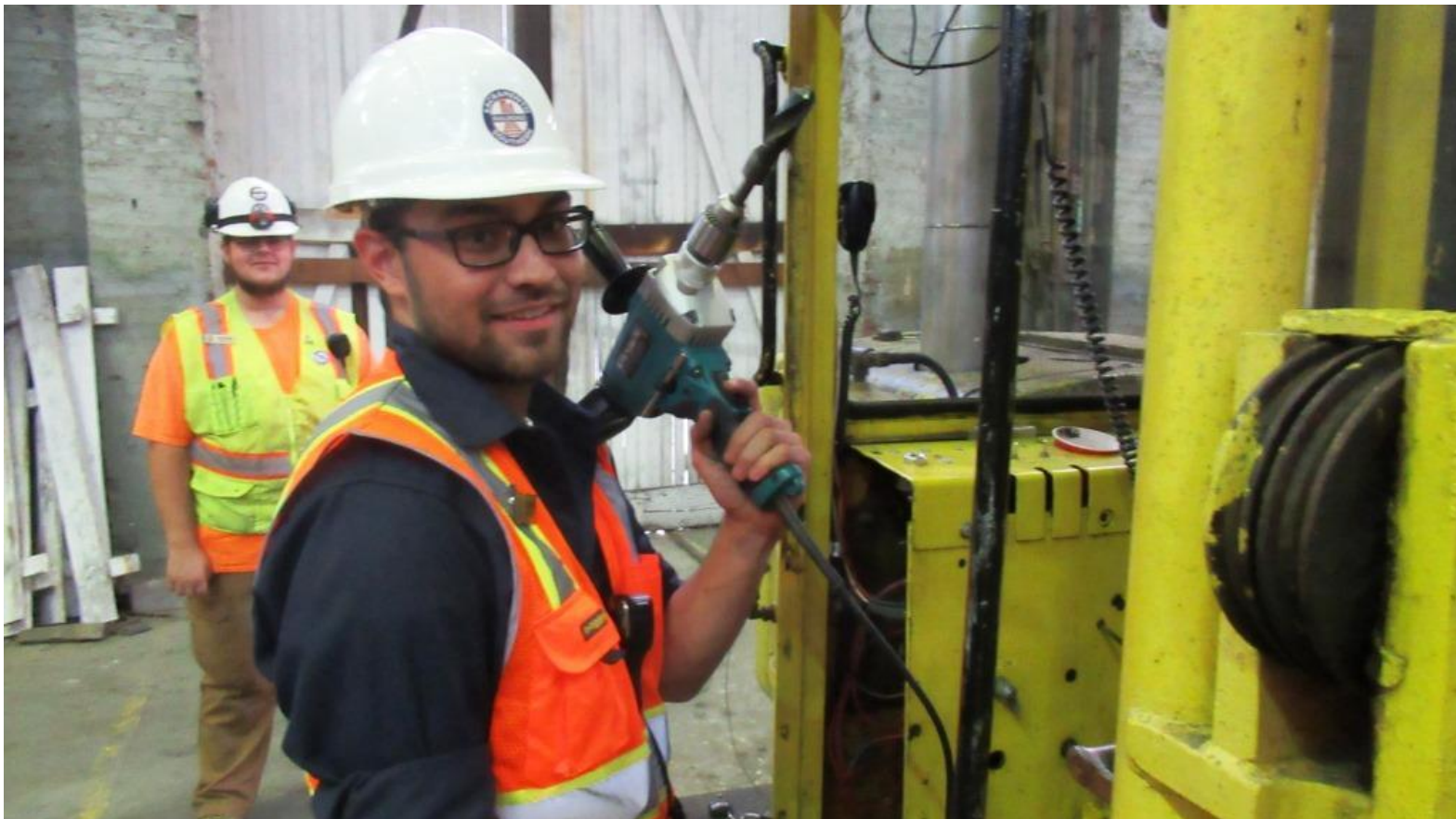
Kyle gets out the big drill to enlarge the hole in the dash of the Kalamazoo to fit a new ignition switch
