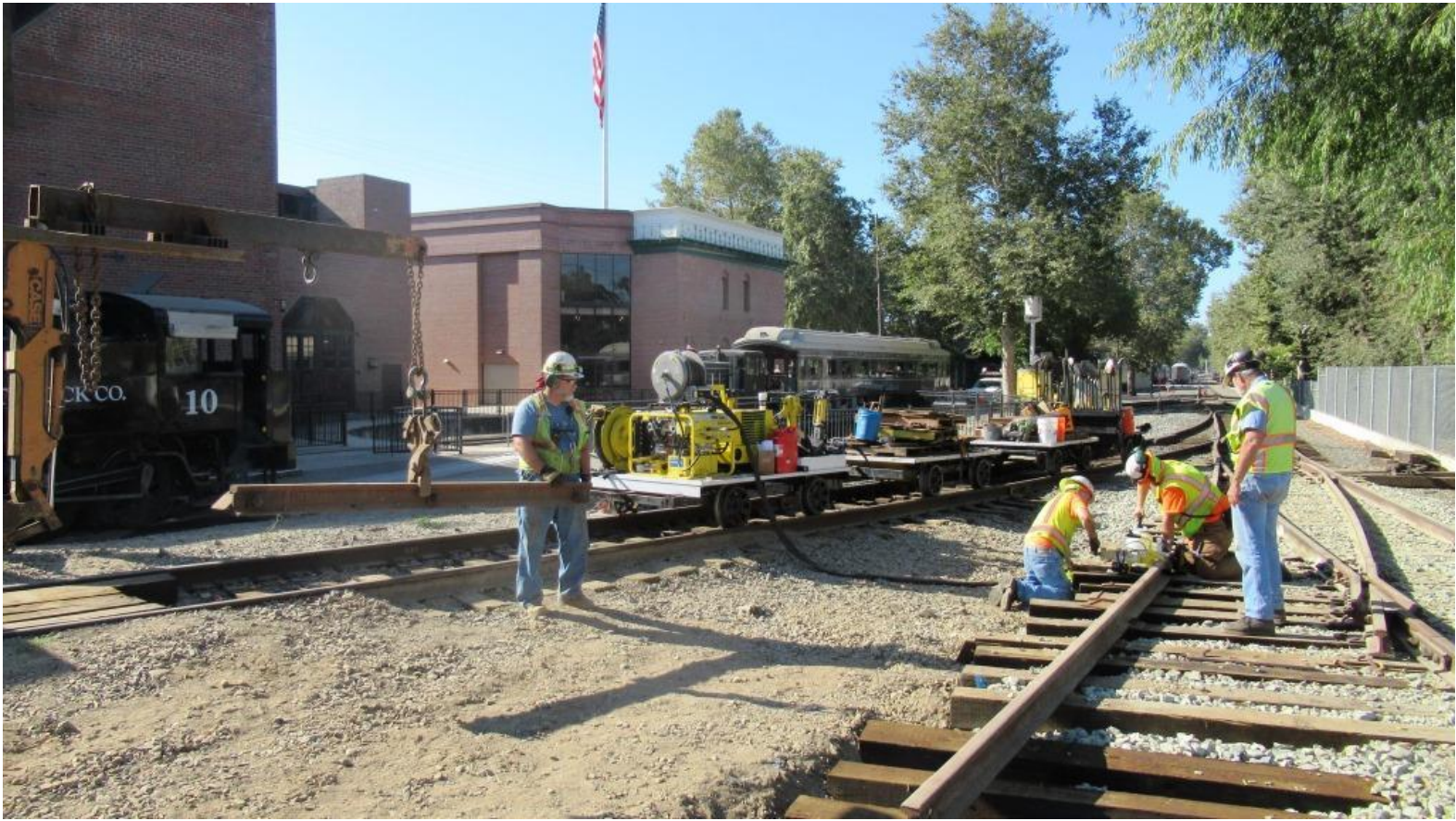
Lots going on in this picture: Granite Rock 10 is being fired-up, the El Dorado is moved on the turntable, Mike F. is ready to place the guard-rail, while Mike H., Chris, and Alan drill bolt holes in the web of the diverging rail
