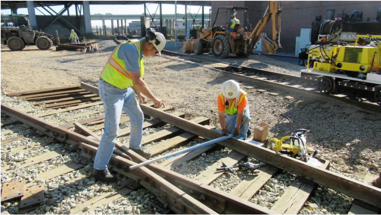
Meanwhile, back in Old Sac., Alan and Mike H. take precise measurements for the placement of the guard-rail
