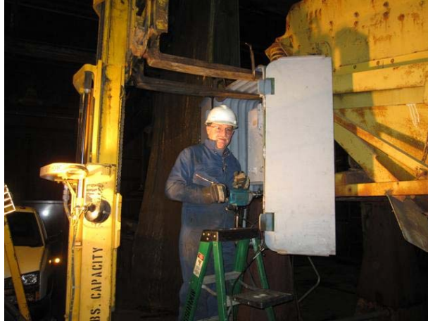
Mike attaching the security box for the electrics to the shaker.
