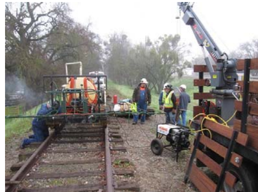
Repairing the Cliff's spray rig. Harry on the welder while the others clean up the equipment.
