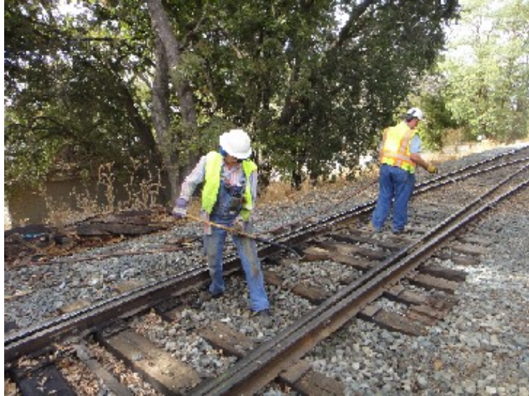
Steve shoveling ballast which Chris uses the air hose to clean leaves.
