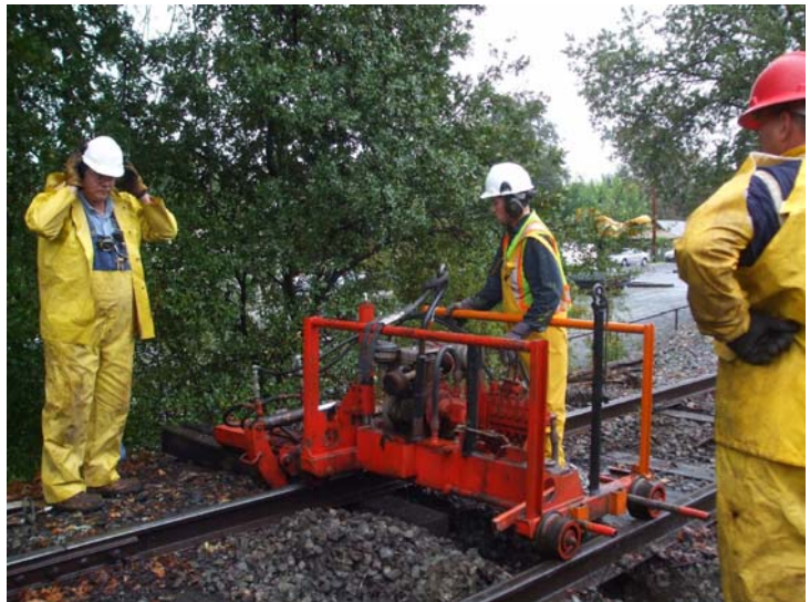
(l-r) Chris, Brenton, and Steve use the Section Gang machine to change out ties at Jamestown.
