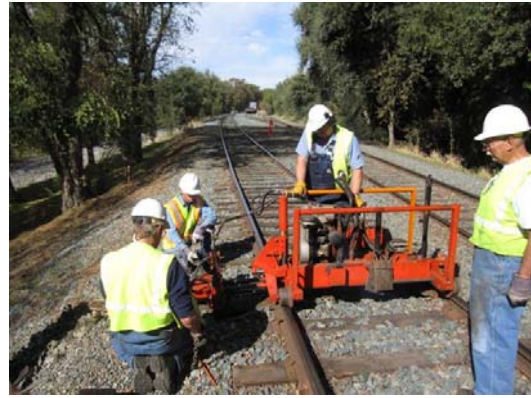
Steve, Brenton, Chris, and Clem using the section gang machine to change ties.
