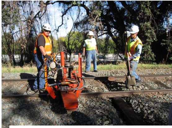
Harry, Clem, and Brenton preparing to insert a tie with the section gang machine.
