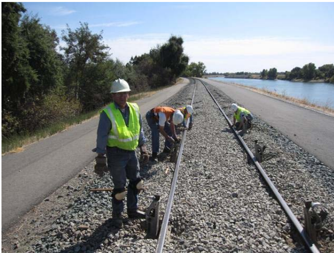
Mike Taylor in front, Steve, Brenton, and Richard setting track jacks for the track raise
