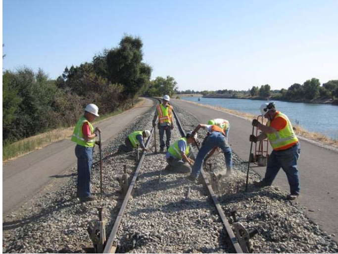
Most of the crew clearing ballast and setting setting jacks for the raise.
