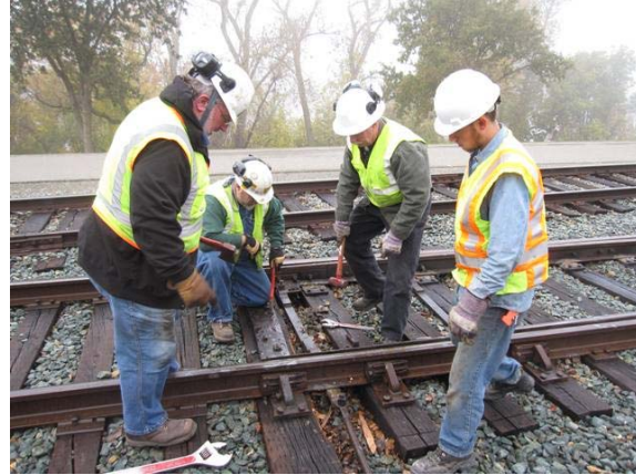
(l-r) Frank, Mike, Ed, and Brenton working on a switch at Baths in the foggy cold weather.
