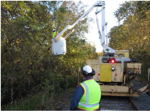
Brenton in the bucket trimming back the trees encroaching on the right of way just south of the I-5 Bridge. Frank looks on ready to move the brush away.
