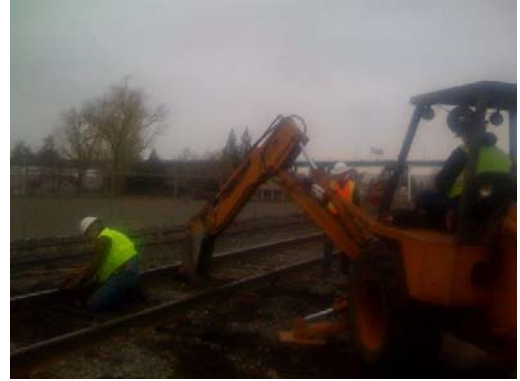
Chris on the Backhoe pulling out a tie while Steve sets spikes on a newly inserted tie.
