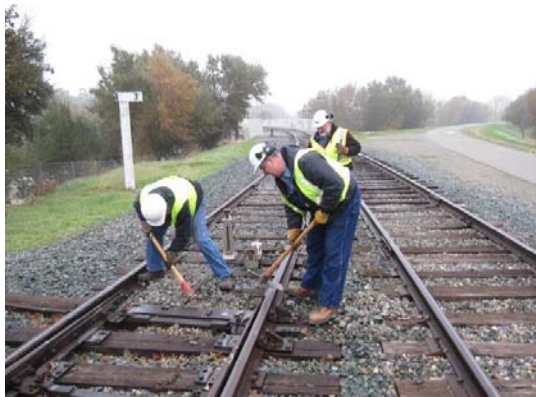
Steve, Chris, and Frank work on switch 19 preparing to move the head block to ease the action of the switch.
