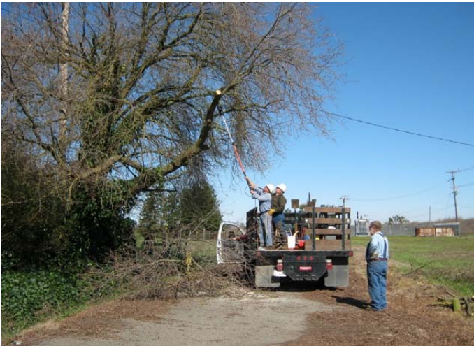
Mike and Joe use the pole saw to clear a tree on the access road to the the Hood yard while Pat stands watch over their safety!
