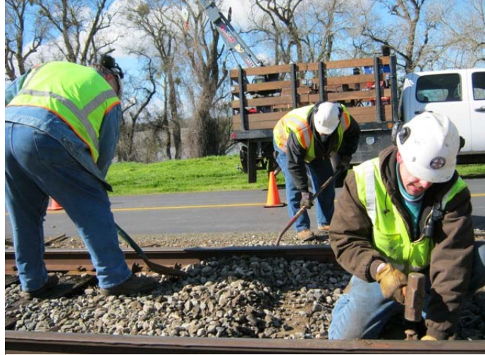
Frank and Chris are shoveling ballast on a newly inserted tie while Richard sets a spike.
