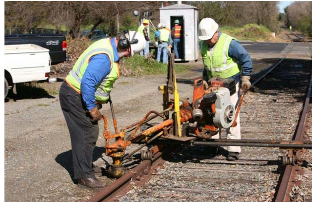
Frank and Jack with the bolt machine tightening the joints south of Sutterville Rd. Signals in the background working on the crossing.
