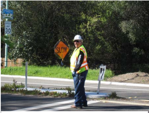
Harry is crossing guard for the day on Riverside Dr. protecting the loader hauling the Pampas Grass to the side dump car.
