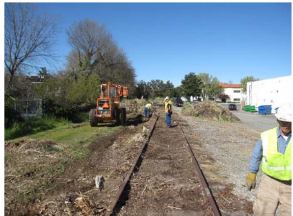
MOW finishing up on the track south of Sutterville Rd. after the Pampas Grass is removed.
