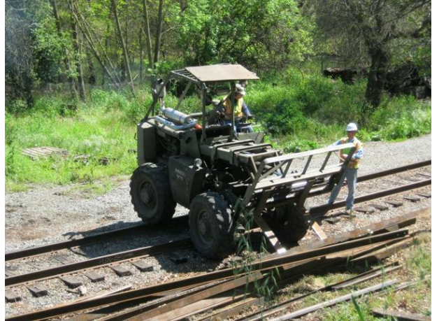
Green machine at Setzer moving rail away from the track to create safe walking space for the train crews.
