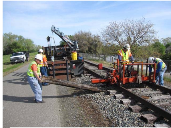
Jack removing the spent tie while Frank and Mike work the Section Gang machine.
