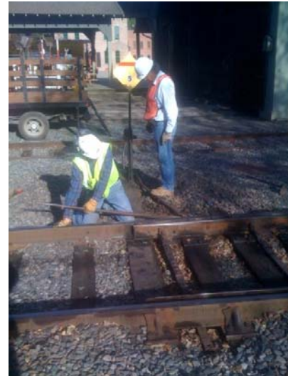
Richard and Ron working on the run through switch in Old Sacramento.
