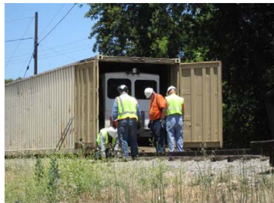
Working on getting the derailed equipment out of the container at Cliffs
