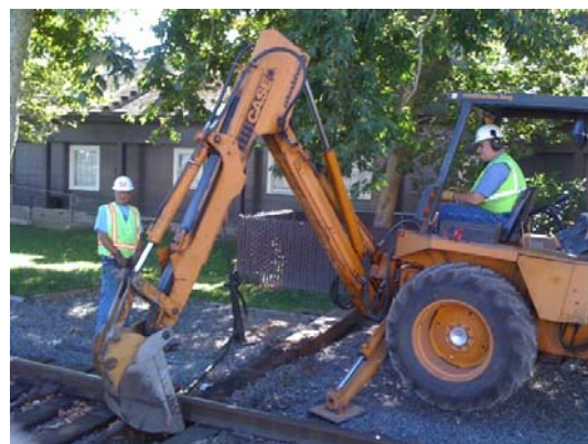
Chris working the backhoe while Jon watches the removal of the old #10 headblock.
