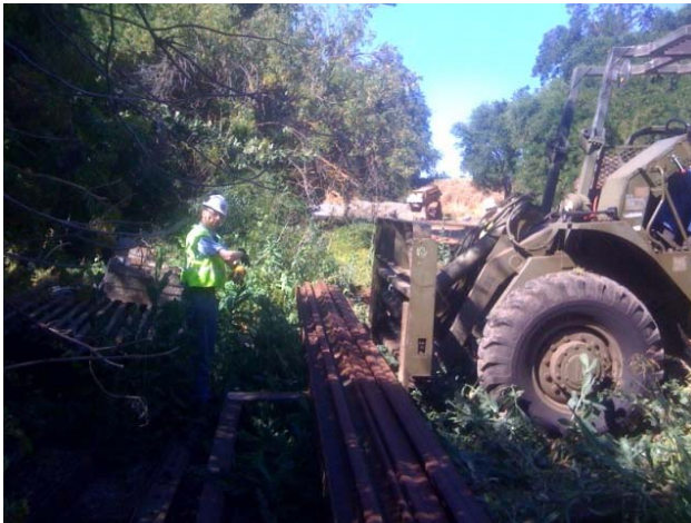
Richard making sure the rail is centered on the ties for safe storage.
