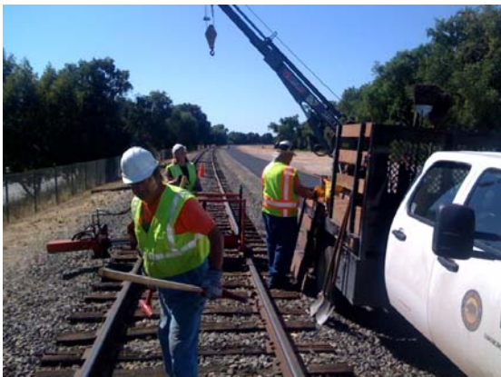
Jon gets ready to drive spikes while Janet and Mike load the section gang machine back on the truck.
