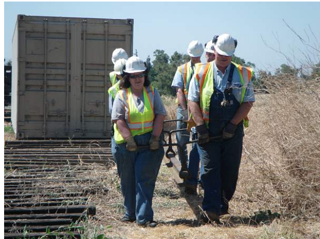
MOW Crew moves rail into position the old fashioned way. That is half a ton of iron they are carrying.
