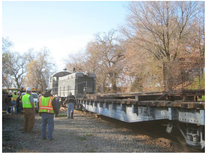
The 2030 moves the flat car with rail down to Setzer as the MOW crew looks on ready to start swarming over the car to unload it
