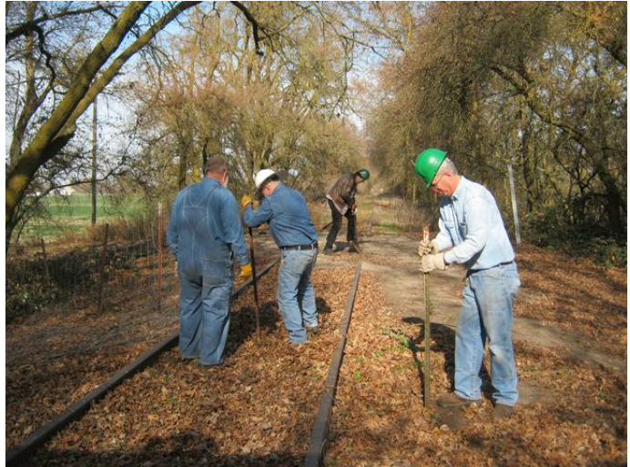
Pat, Joe, Randy, and Dave work on clearing the Hood line at the south crossing.
